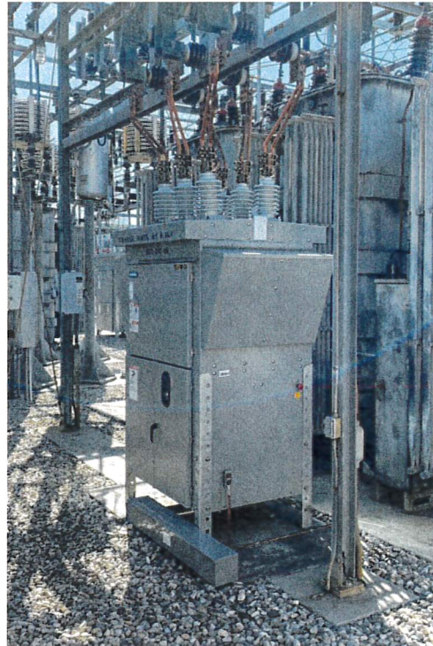
New Transformer A-1 MV VCB
