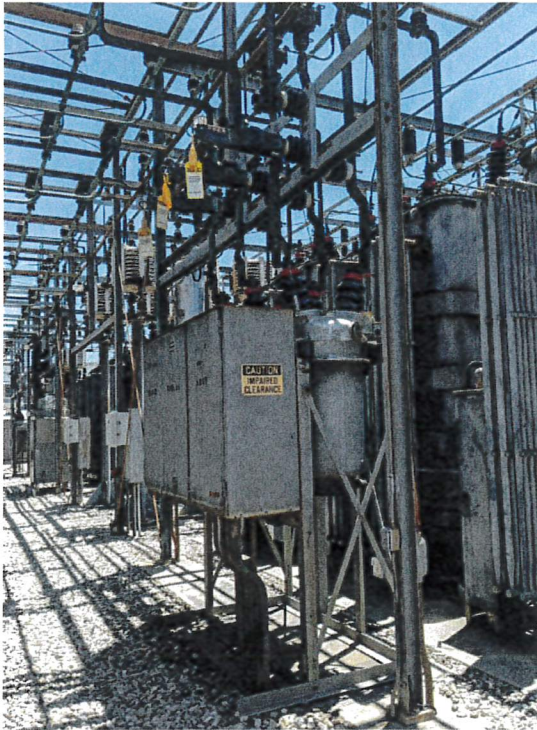
Old Transformer A-1 MV OCB
