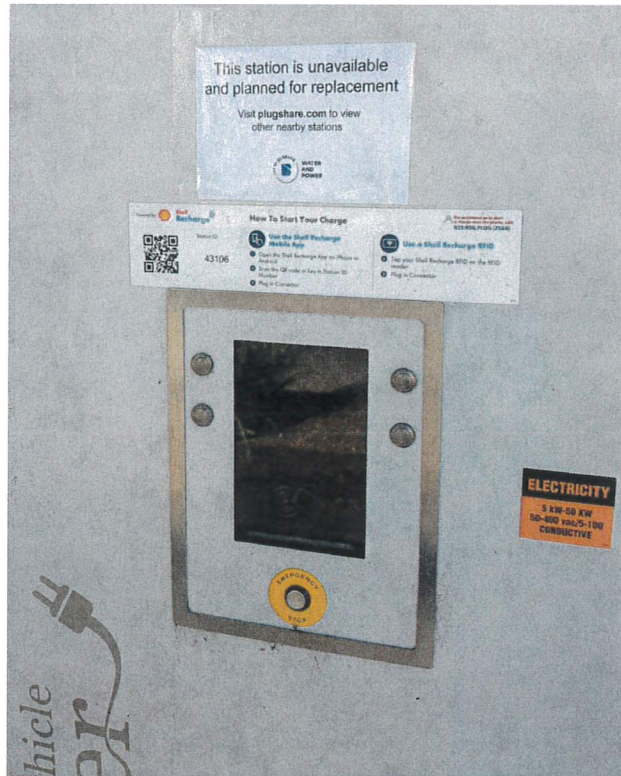
Signage placed on non-operational DCFC at Lakeside Shopping Center.
