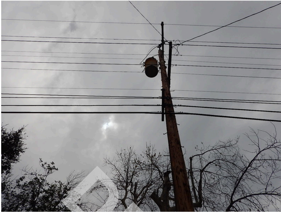
11. View of pole-mounted transformer at subject property
