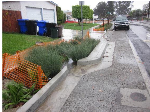
Example of bioretention and permeable pavement retrofits during construction, San Diego, CA
