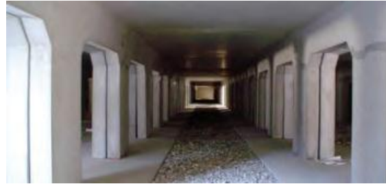
Example subsurface infiltration gallery (source: City of Los Angeles)
