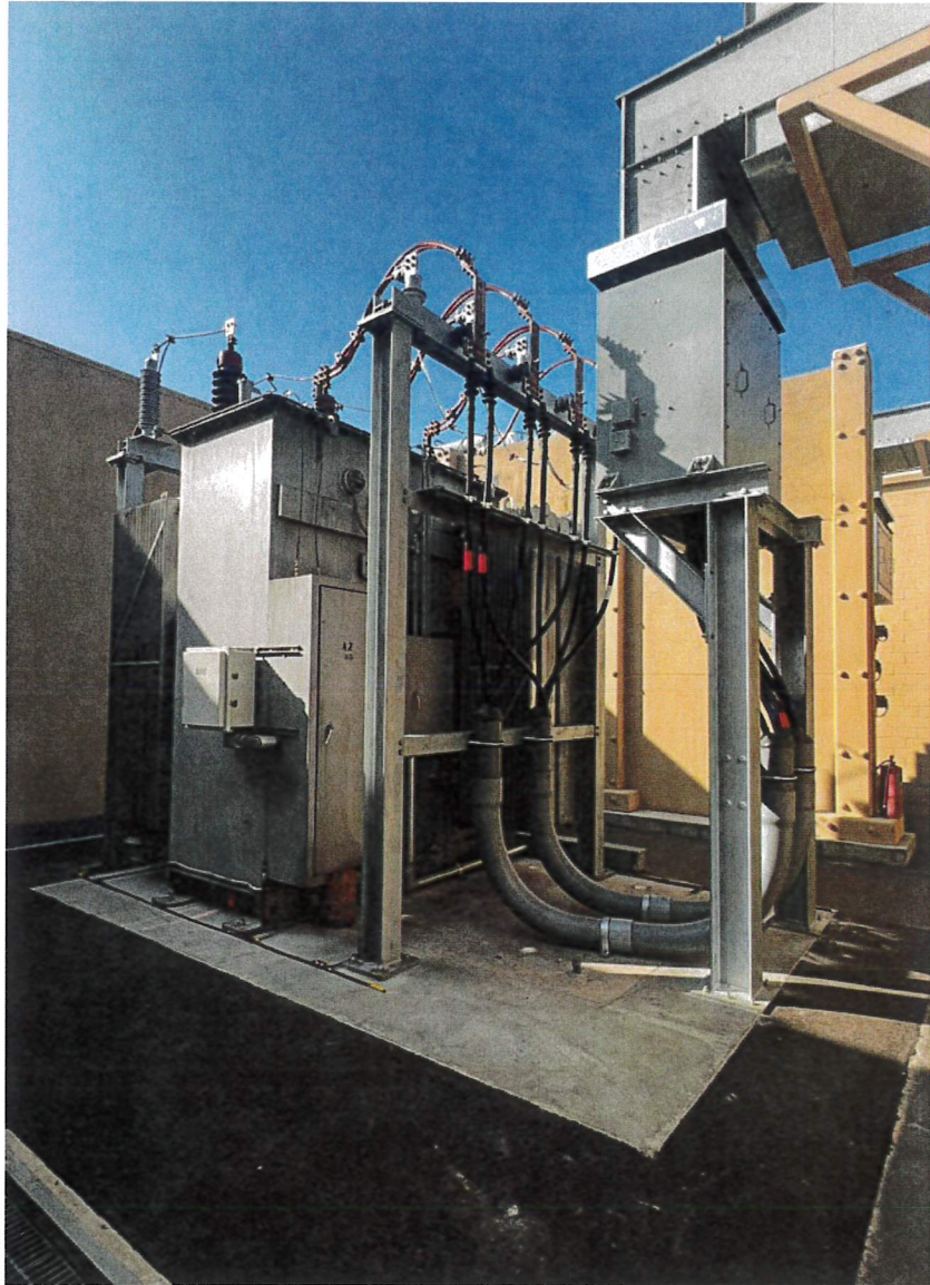
Temporary Transformer at Warner Customer Station
