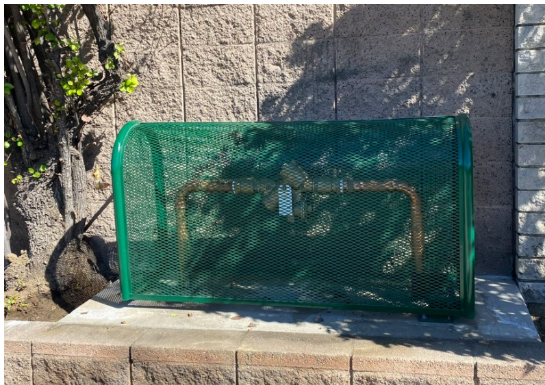
Backflow Device @Town Substation
