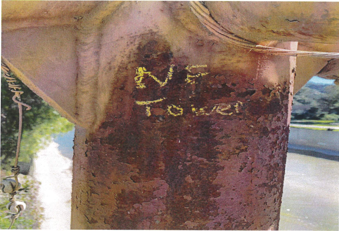
Photo 7_Examples of Surface Rust on all Four Towers
