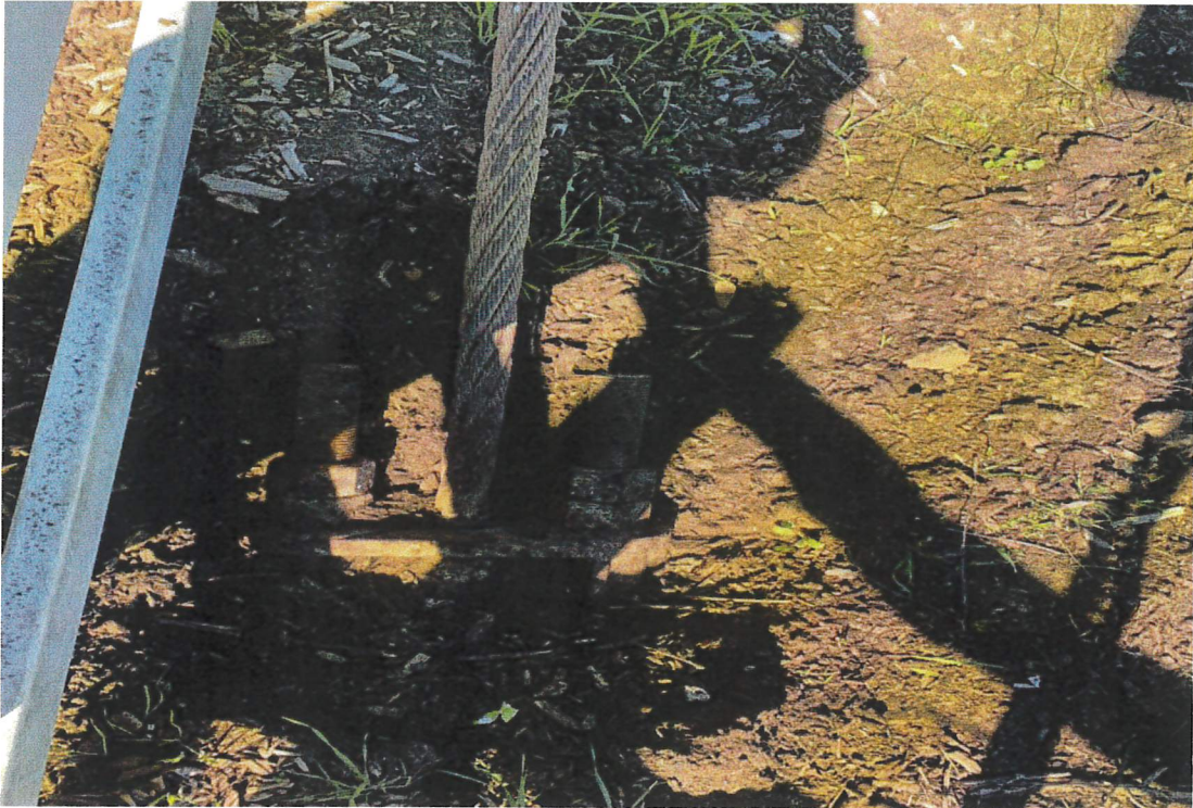
Photo 10_Surface Rusting at Suspension Cable Anchor Points
