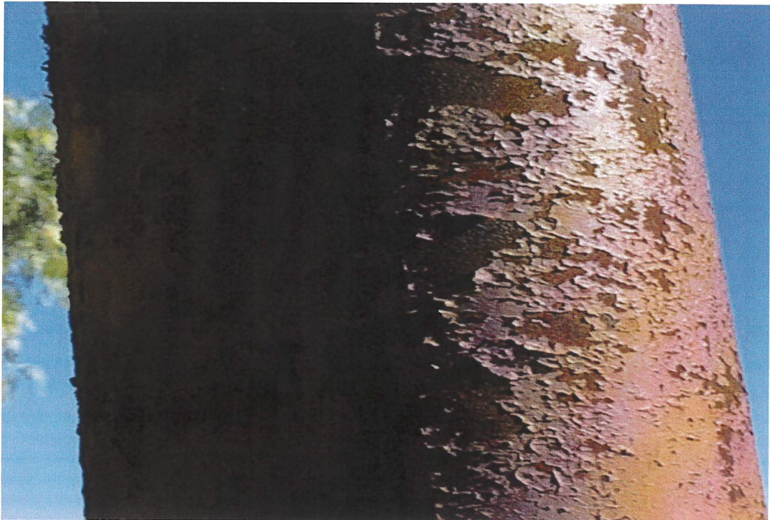
Photo 8_Flaking Rust Examples
