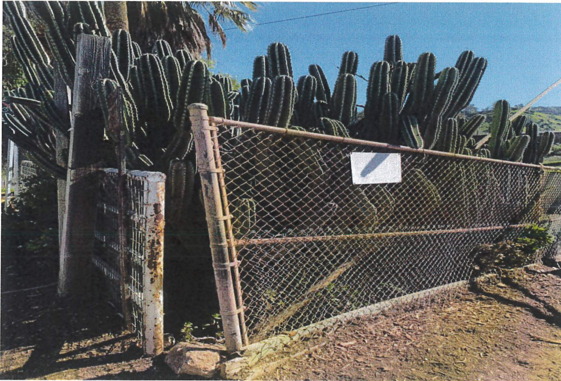
Photo 3_Entry Gate Needed at NorthEast Suspension Cable Area for Inspection
