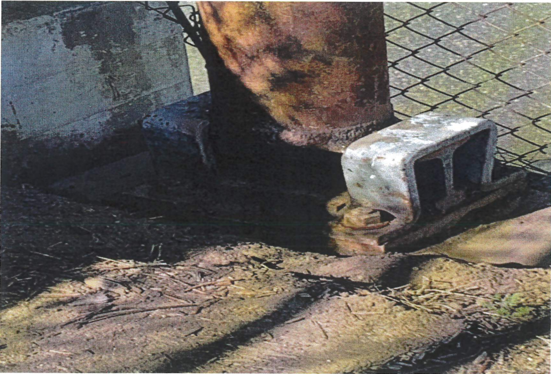
Photo 9_Rusting at Tower Columns Anchor Points
