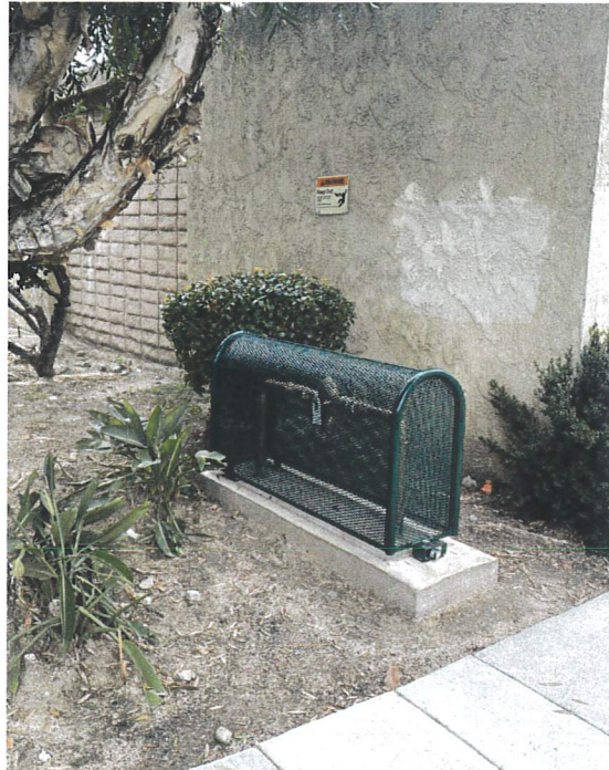
Backflow Device @San Jose
