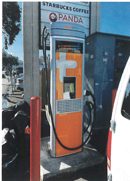
New DCFC at the Lakeside Shopping Center
