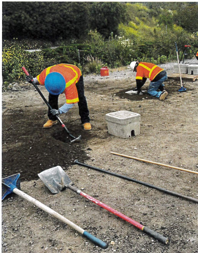
Candidates shown here are utilizing various tools to install a water meter box.
