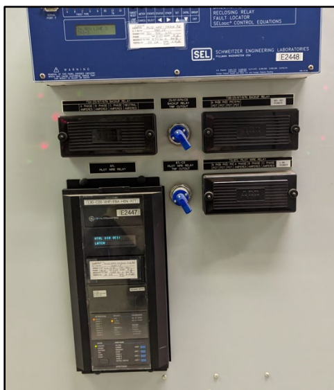
Before Installation (Old Relay)
