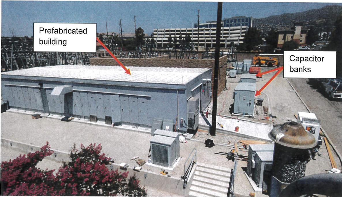
Prefabricated building and Capacitor Banks Delivered
