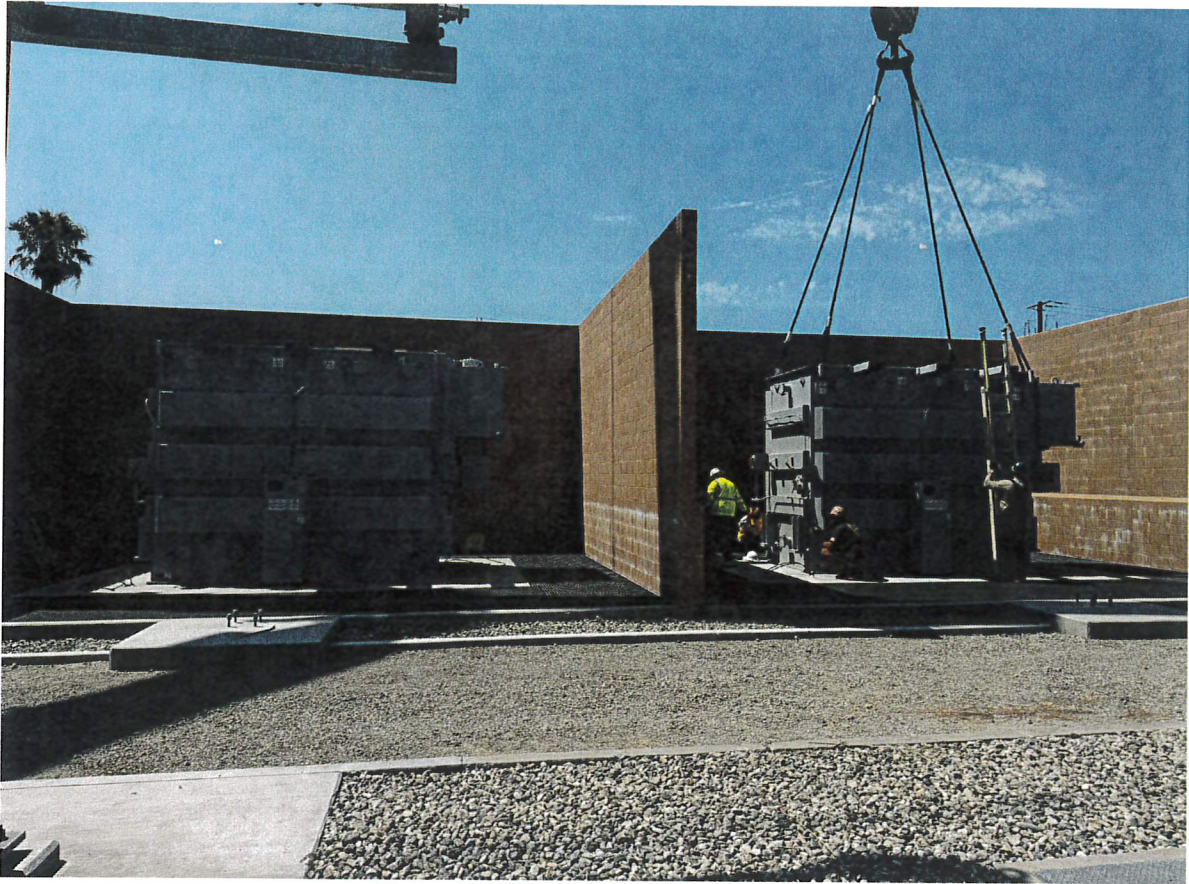
Power Transformers Delivered Onsite
