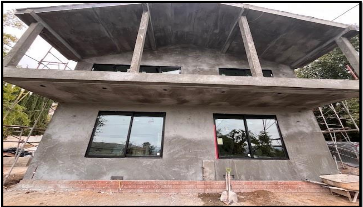
Figure 10: View of the existing front façade from the south portion of the property where the proposed first floor front porch will be constructed.
