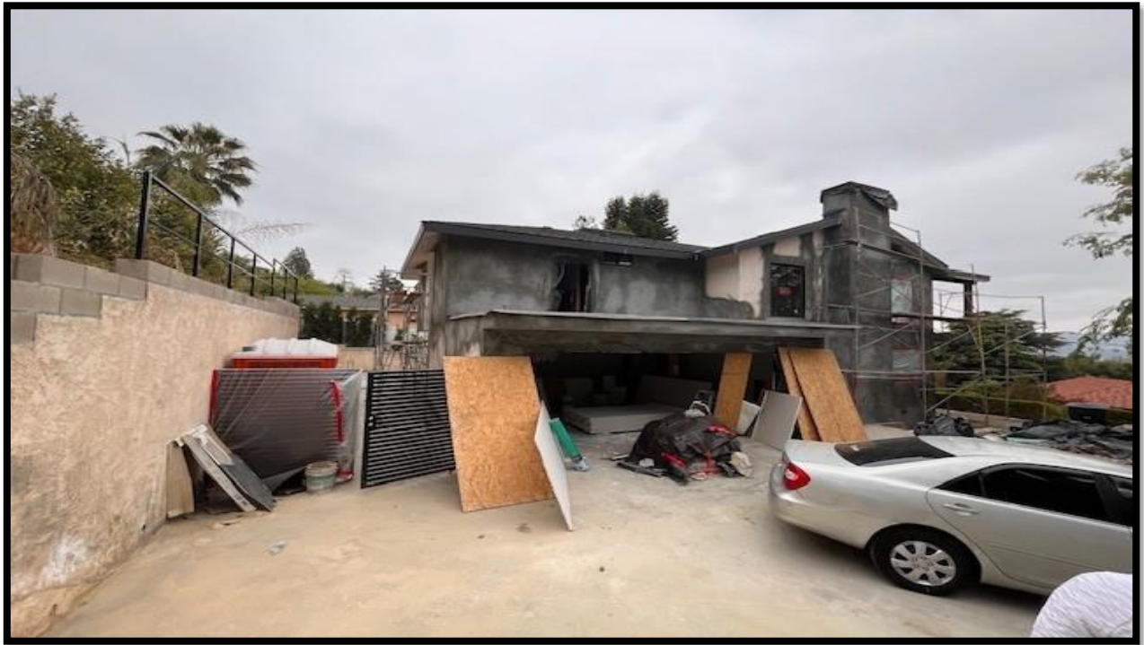
Figure 9: View of the existing residence from the northwest portion of the property where the rear porch will be constructed.
