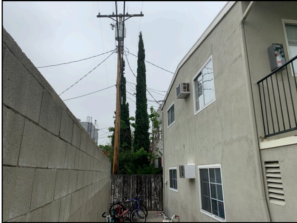
Photo 2: View of pole-mounted transformer located immediately adjoining to the northwest portion of the subject property.
