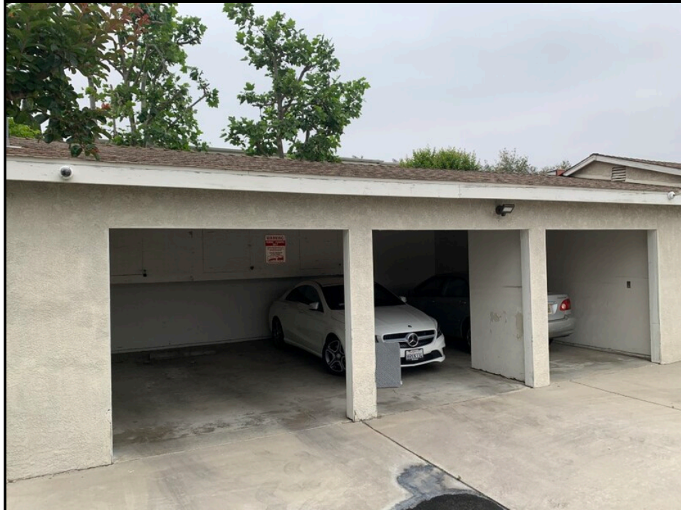
Photo 12: View of carport located west of 2333 North Fairview Street looking to the north.
