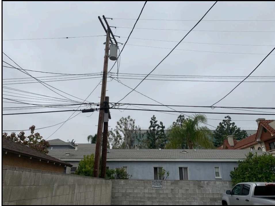
Photo 22: View of pole-mounted transformer located immediately adjoining the southwest portion of 2321 North Fairview Street.
