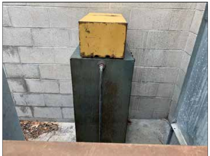
24. Emergency generator diesel day tank
