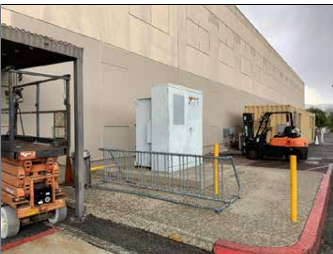
29. Transformer on south side of Convention Center
