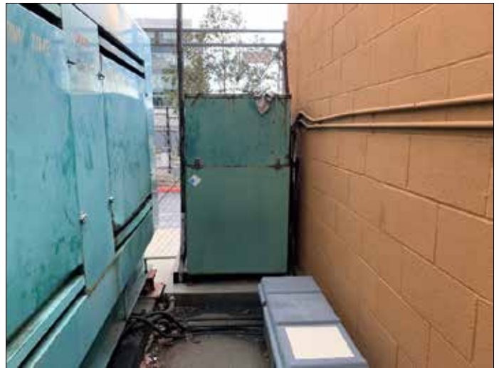
22. Emergency generator diesel day tank
