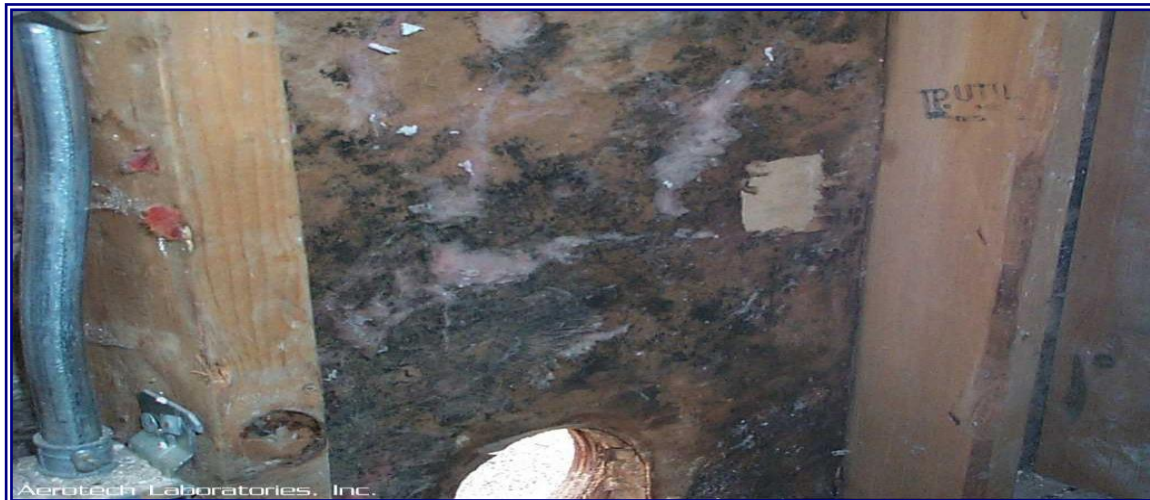
Photo of mold growth that was hidden beneath insulation inside the wall cavity.
