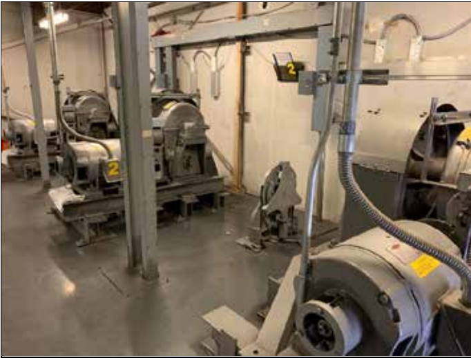
19. Elevator equipment in West Tower
