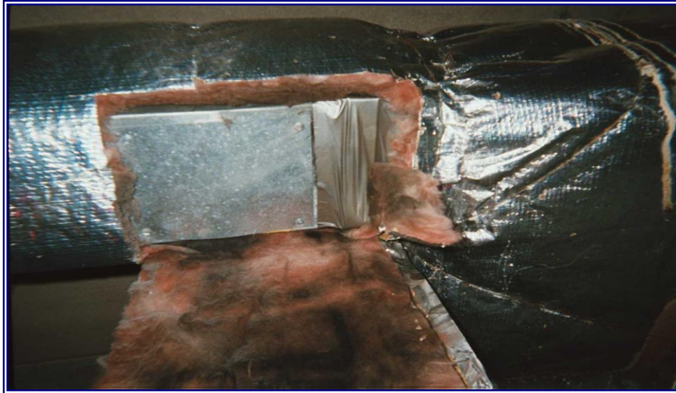
Photo of insulation that was routinely wet by condensation and became a growth site for black mold.
