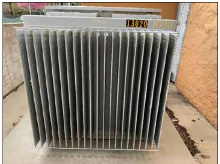
28. Transformer on south side of hotel
