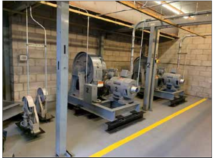
20. Elevator equipment in East Tower
