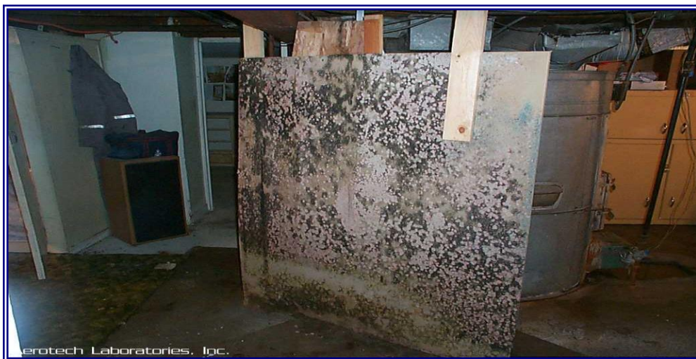
Photo of a basement partition where water damage was affecting a limited area of the basement and was allowed to go unchecked until the mold bloom was investigated
