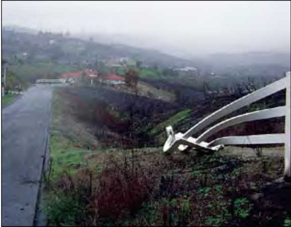
Figure 2. Plastic fences can melt even under moderate wildfire temperatures (FEMA field team).
