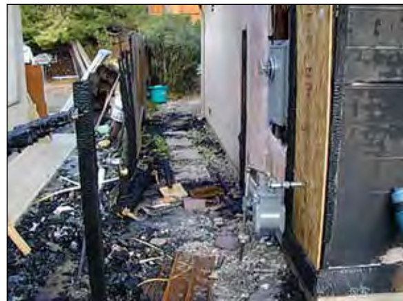
Figure 1. The gate that was attached to the garage at the corner ignited and led the fire to the home, causing the damage seen here ( firecenter.berkeley.edu ).
