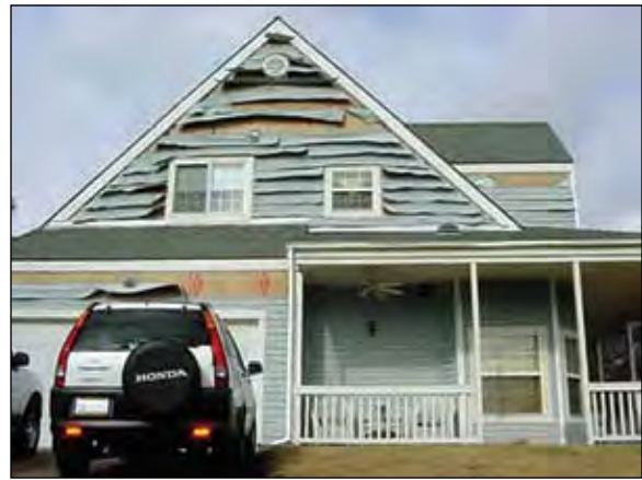
Figure 1. Vinyl siding that melted and warped during a wildfire (firecenter.berkeley.edu).
