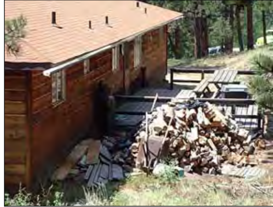
Figure 2. Combustible materials adjacent to a building create a hazard (Anchor Point Group, Boulder, CO).
