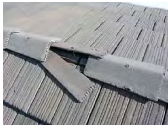
Figure 3. Displaced tiles allow ember entry.
