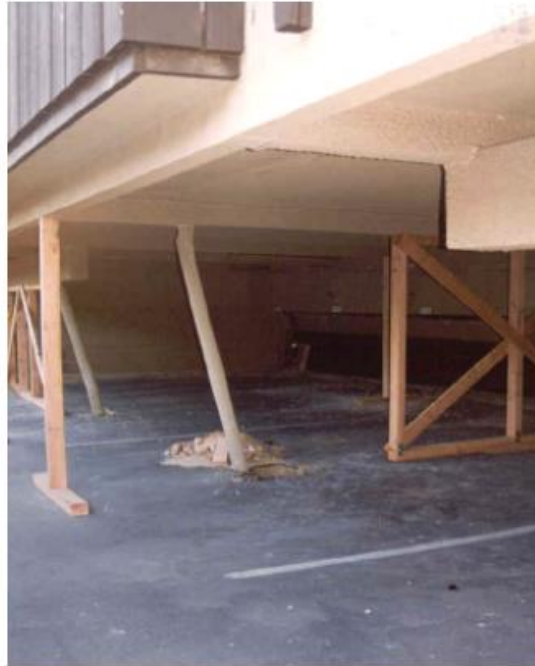
Figure 1-7 Northridge Gardens apartment building following the Northridge earthquake with direction of drift perpendicular to the open front (image credit: Schierle, 2003).
