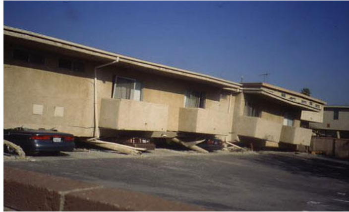
Figure 1-3 The Northridge Meadows Apartment building, representative of a long-side-open SWOF building type with a collapsed weak and soft story (image credit: Robert Reitherman, CUREE).
