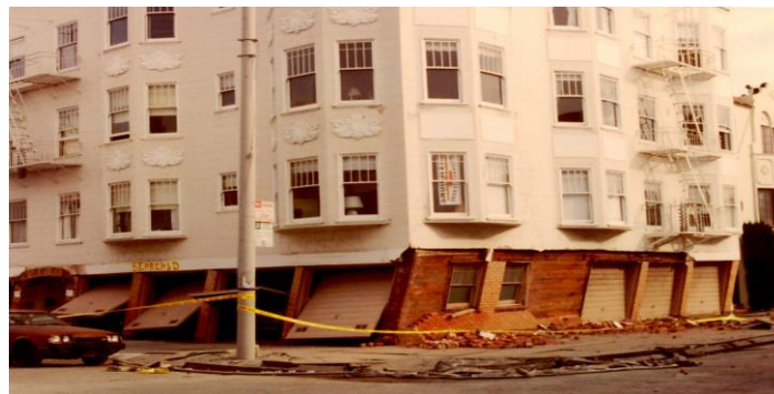
Figure 1-5 SWOF building with both sides open in the San Francisco Marina District showing weak-and-soft story behavior (image credit: Ron Gallagher).
