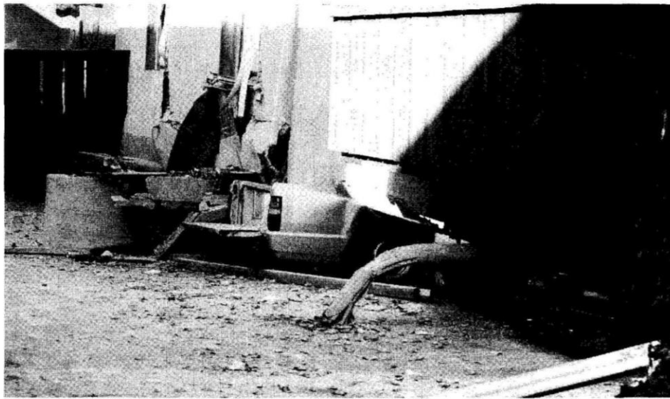
Figure 1-6 Apartment building following the Northridge earthquake with a collapsed column showing direction of collapse perpendicular to the open front (image credit: EERI, 1996).
