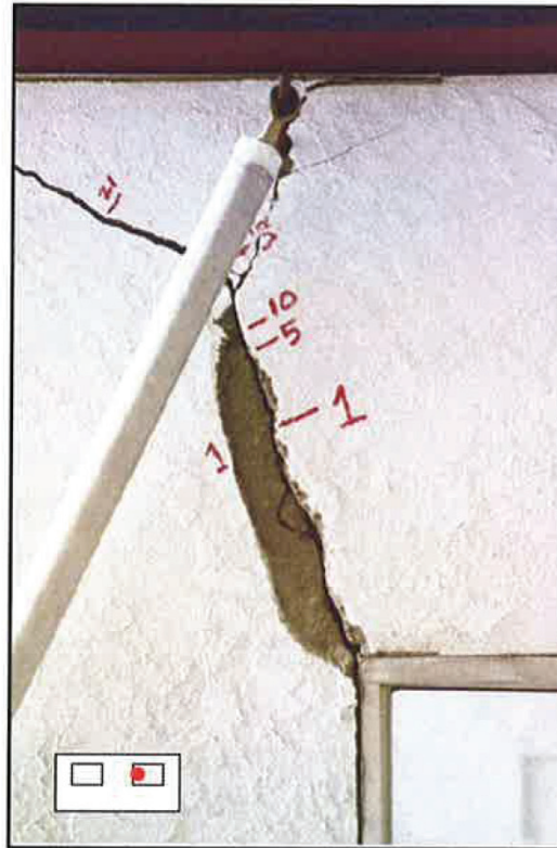
(b) Finish Coat Spalling
