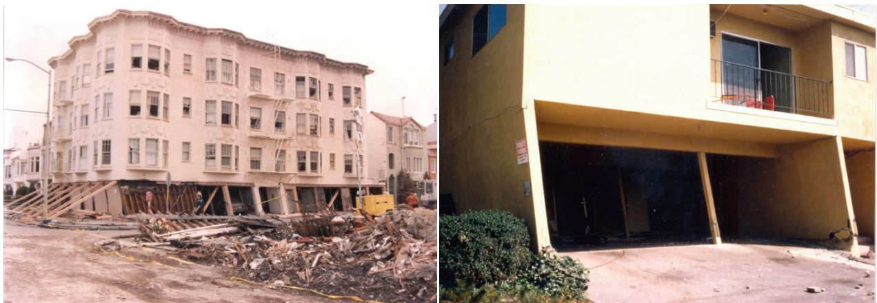
Figure 1-1 Photos illustrating near-collapse of typical weak-story wood-frame buildings in the 1989 Loma Prieta earthquake (left) and the 1994 Northridge earthquake (right).
