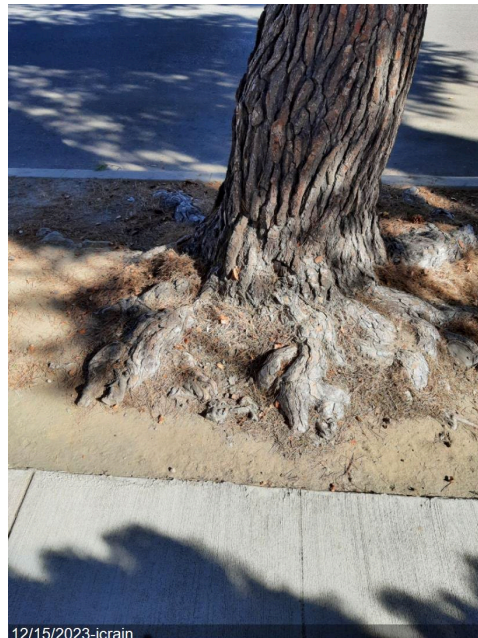
Previous root cuts 18" from trunk.
